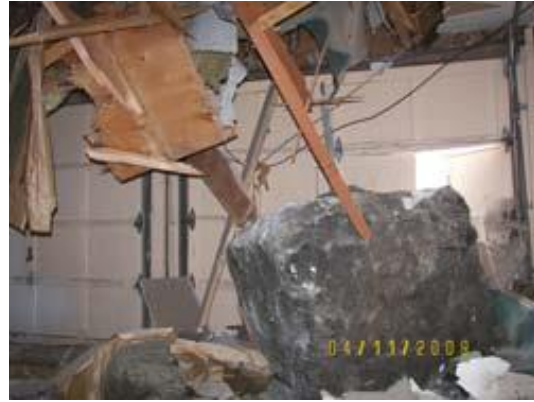
Boulder that damaged the vacant house at 1496 North 1550 East, Provo. Boulder is estimated to be 4x5x4 feet. Photo courtesy of the Provo Fire Department.
