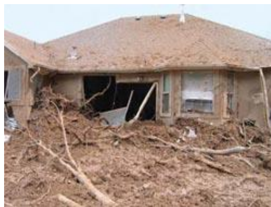
The rapidly moving landslide that slammed into this house at 7687 South 1650 East, South Weber, broke through the back wall and injured a child inside.
