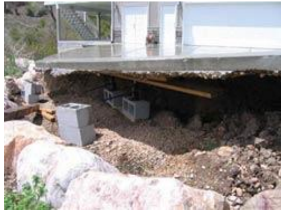
Landslide movement left this concrete driveway slab suspended in the air in the Creekside Drive area, Mountain Green.
